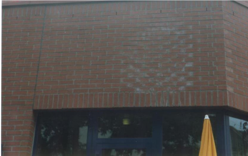
Figure 4: Salt efflorescence on the wall surface 4
