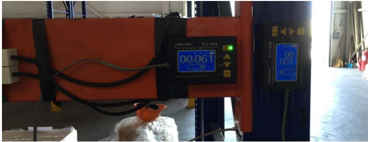
Figure 5. Inclinometer located within the beam-to-column connection
